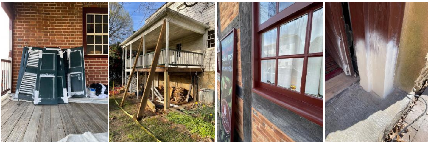
(left to right) Winkler Bakery Shutters; Blum House Porch reconstruction; Fourth House Main Street windows; Fourth House door jamb reconstruction
