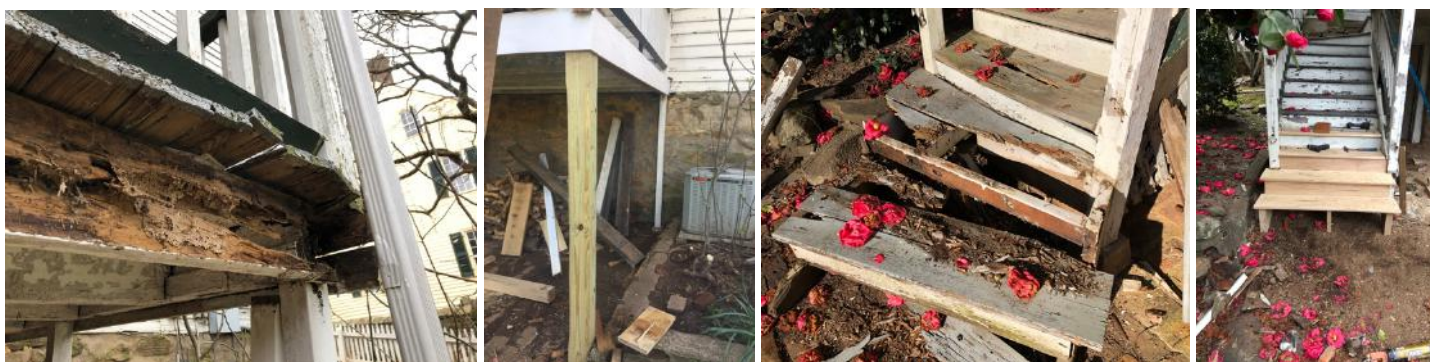
(left to right) Blum House rear porch structure deterioration; Stair rot; Repaired stair; Repaired porch structure.
