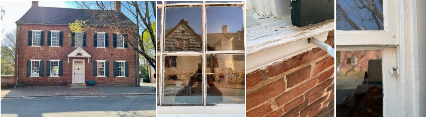
(left to right ) Vogler House is set to get all of its windows and doors restored. We made public an RFP process to chose a contractor to facilitate this work. As part of our EQUITY INITIATIVE, we are expanding our outside vendor list. The goal of this Vogler RFP is to restore the windows to operability.
