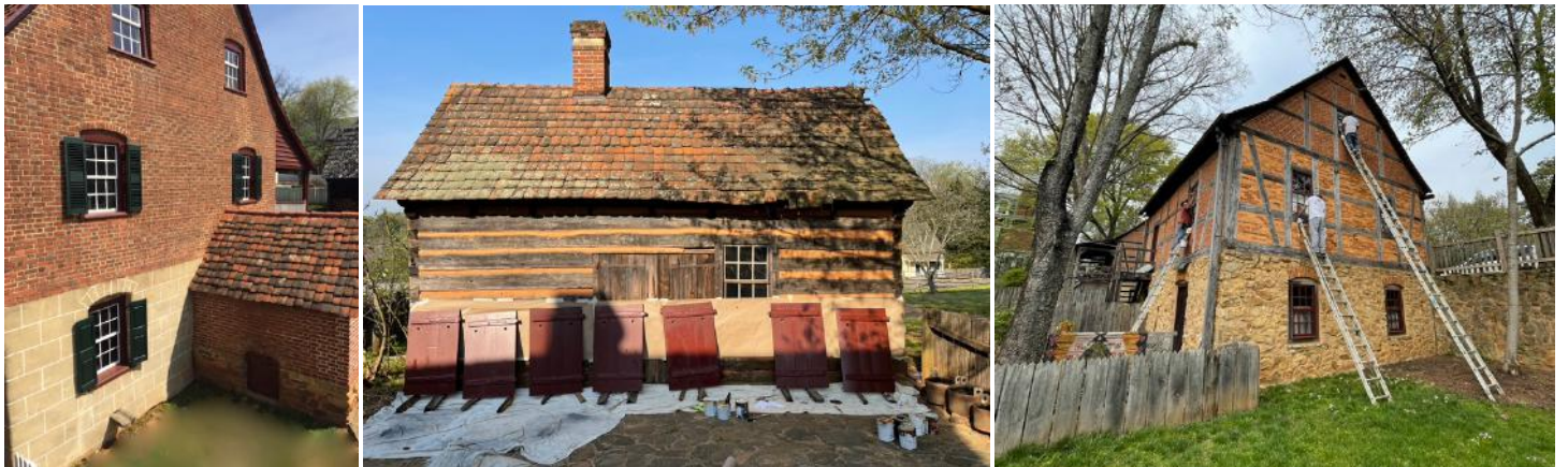
(left to right) Winkler Bakery South facing shutters repaired & re-installed, Miksch House shutters repaired (one newly crafted) and painted, The Fourth House gets TLC.
