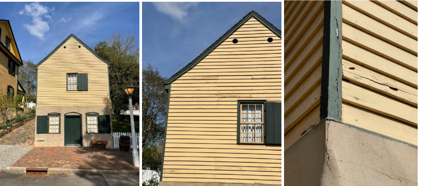
(left to right) The Hat Shop (The first jail of Salem) has minor wood repair and in need of repainting. This building will be our next Fresh Coat Initiative project.
