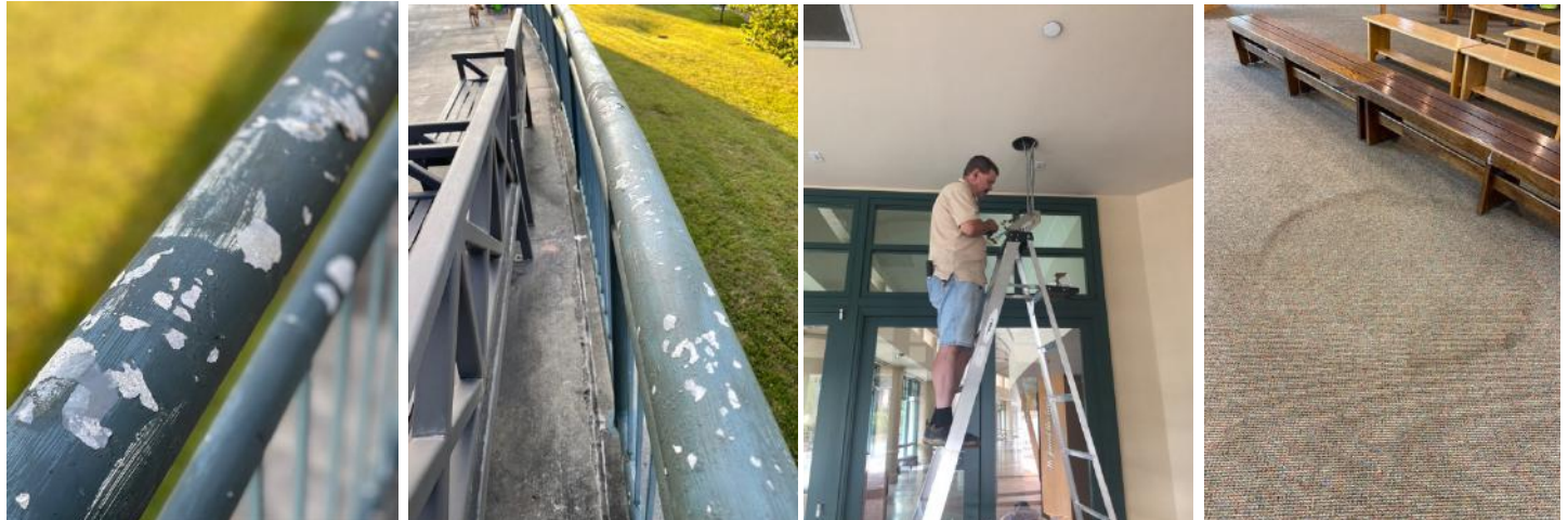
(left to right) The extensive upper loggia railing is getting prepared and repainted. In preparation for our Phase Two Reopening, Tony Bragg, Facilities Team Member , replace light fixtures at the Visitors Center. Thank you to our Facilities Director, Erik Skarzynski , and Director of Community Engagement and Visitors Center, Samantha Smith , for managing these (and other fresh coat) projects at the VC.
