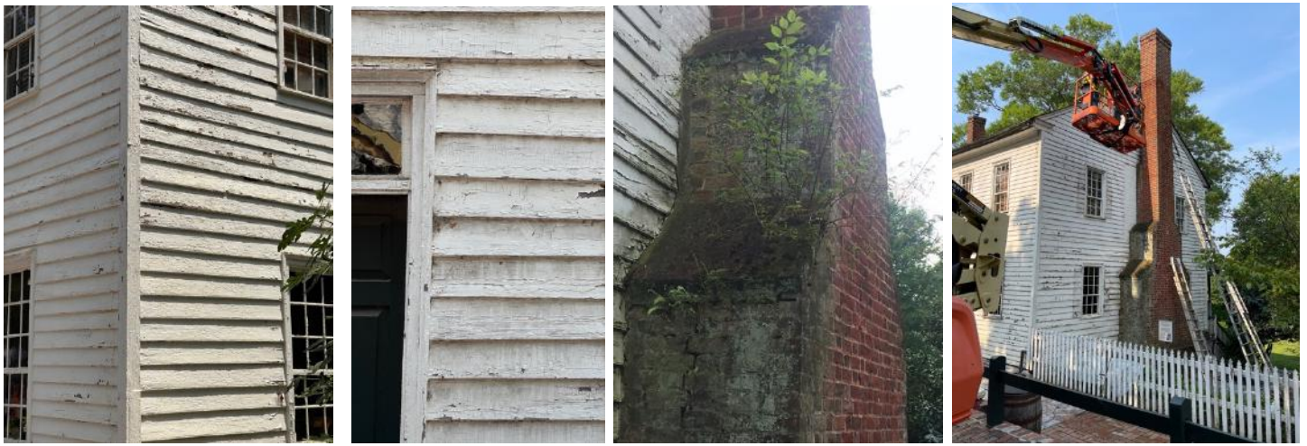
(Left to right) The exterior condition of the Blum House had significantly deteriorated. Because of its massing, a lift was needed to prepare and repair building fabric on the upper levels of the house. The first step in preparing the home for repairs was to delicately wash the house and chimney. Care was taken to follow preservation best practices to avoid infiltrating wood siding or introducing moisture to the historic bricks which could cause spalling.
