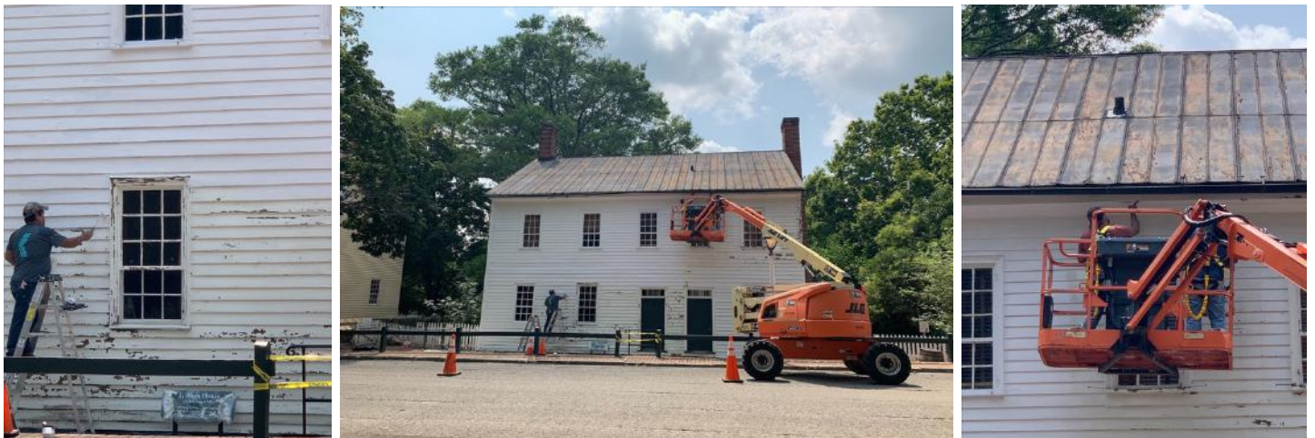
(Left to right) The preparation process for the exterior repainting of the Blum House was involved. First, careful placement of plastic tarps around the building allowed us to capture debris. Next, the thorough, careful cleaning of the entire exterior revealed areas where wood repair was needed. After the necessary wood repair, our wonderful painters carefully scrapped and primed the exterior and applied several coats of fresh paint.
