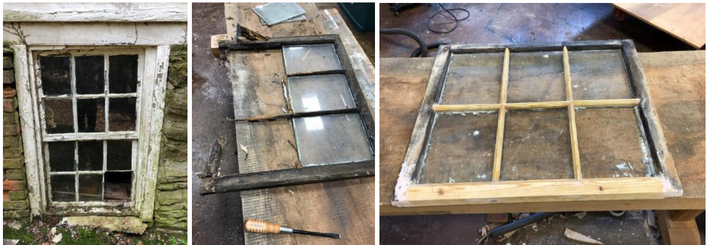
(Left to right) Before any repainting could occur, we had to assess the restoration needs of various building parts. Shown above is the condition of one of the basement windows that needed extensive repair and restoration. The restoration of the wood sash was primarily completed by joiner Ben Masterson with the logistical assistance of Erik Skarzynski , Director of Facilities.
