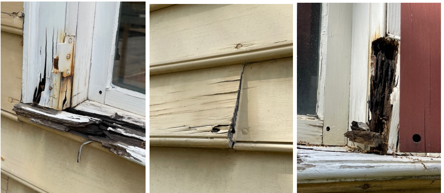
(Left to right) The exterior wood sheathing and window frames needed some level of repair or replacement. The sills had become so rotten that the shutter hinges had fallen free from the screws and the shutters were poorly attached. As you can see from these photographs, the repairs needed to take place before any Fresh Coat Initiative painting could be done.
