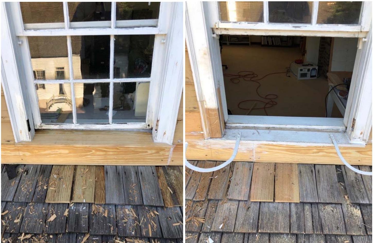
(Left to right) Joiner Ben Masterson completed the expert repairs and restoration work with the logistical assistance of Erik Skarzynski, Director of Facilities. These types of restorations are like infill puzzle pieces carefully inserted into pre-existing building material.
